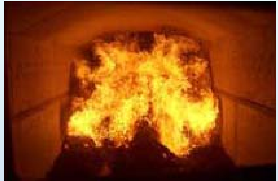
Combustion Unit in Operation
